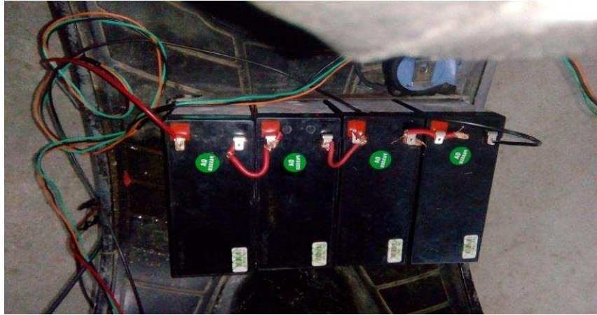
Figure 3: Battery (When Connected)
